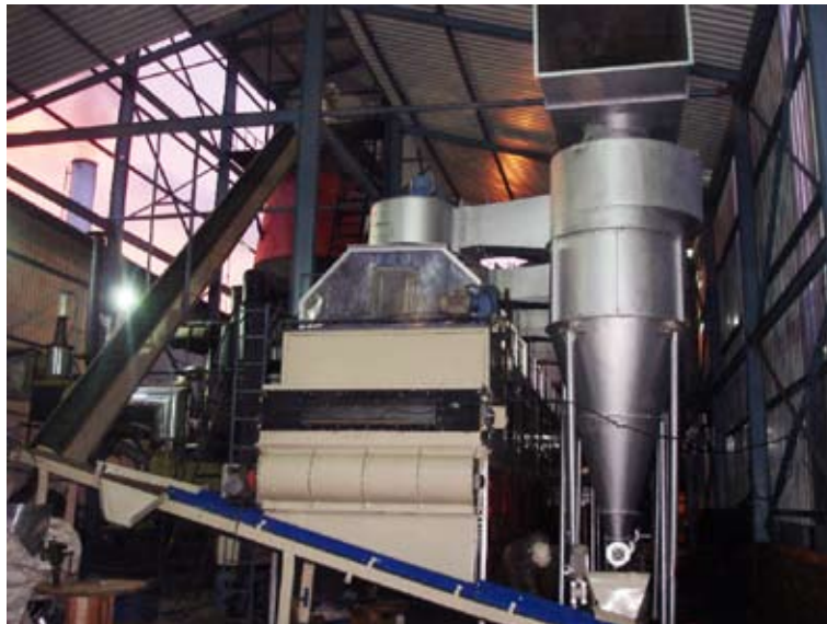
Bio-Gasifier Plant at Instant Tea Operations, Munnar
