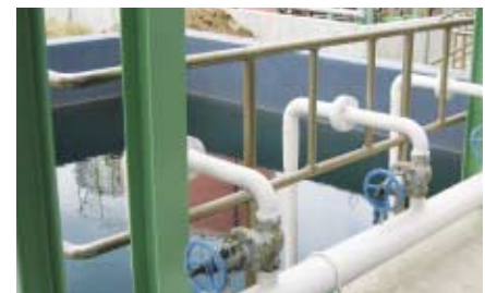
▶ Nitrogen removal facility
