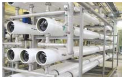
▶ Reverse Osmotic facility
