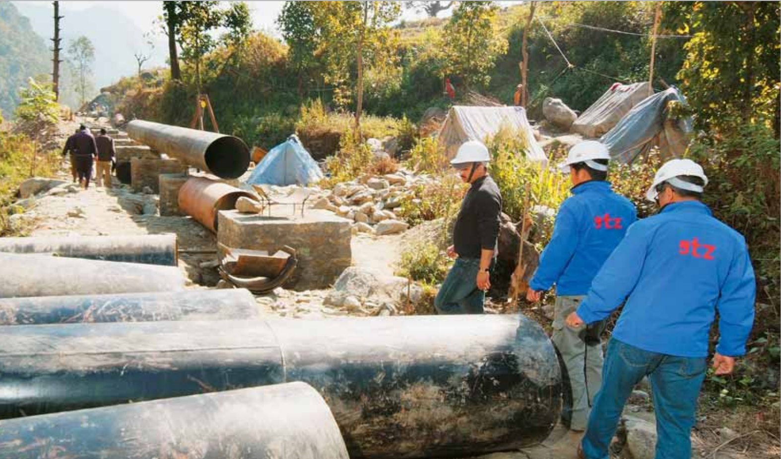
In the pipeline: Shankar Johsi of the Himalayan Bank along with Ajoy Karki and Man B. Rai (both GTZ) inspecting the construction site of the 1 MW hydropower plant "Pati Khola" in Parbat district.
