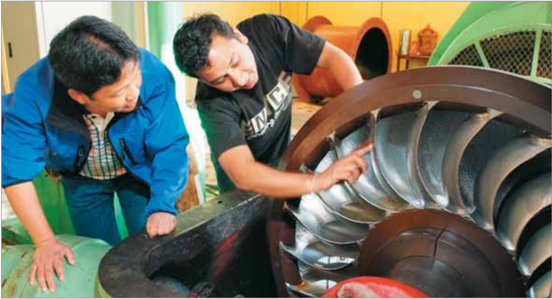
Maintenance required: Bishnu Vantana, deputy manager of the Sun Koshi power plant, showing Man B. Rai of GTZ deposits on the power plant turbine.
