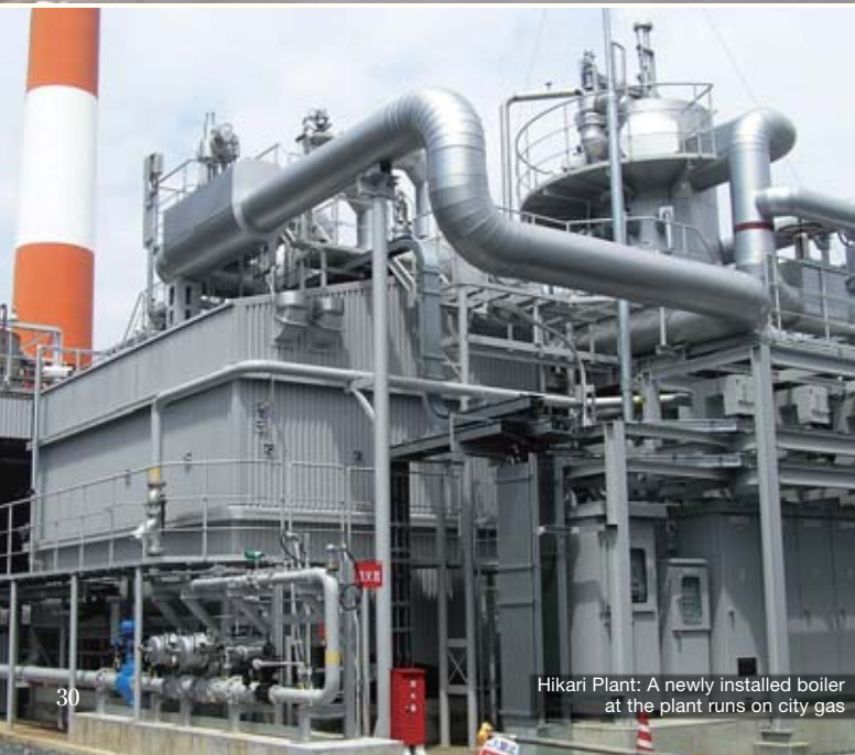
Hikari Plant: Overlooking the Seto Inland Sea the Hikari Plant seeks to coexist in harmony with the environment.
