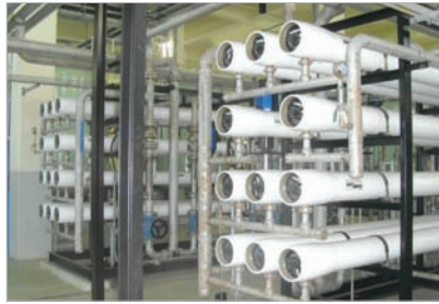
▲ Wastewater reclamation and using system
