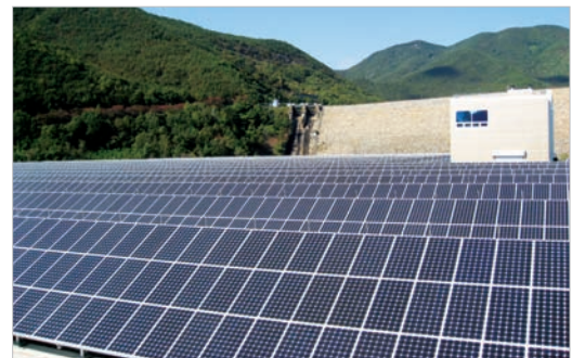
▲ Samrangjin Solar Photovoltaic Power Plant
