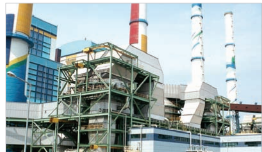
▲ Flue gas desulfurization (FGD) facilities
