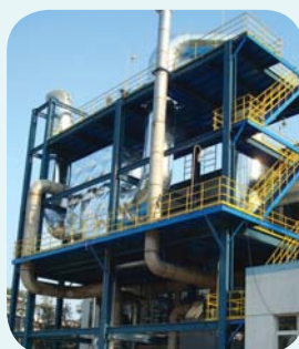
30,000Nm 3 /h rubber exhaust gas catalytic combustion processing installation
