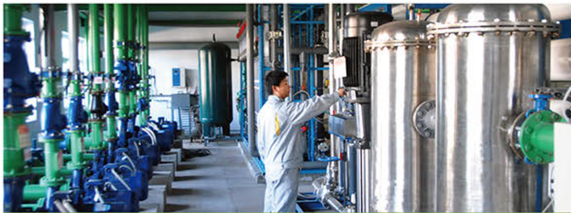
中钢耐火镁质分厂节能环保高温隧道窑 Steel refractory magnesia factory energy saving temperature tunnel kiln
