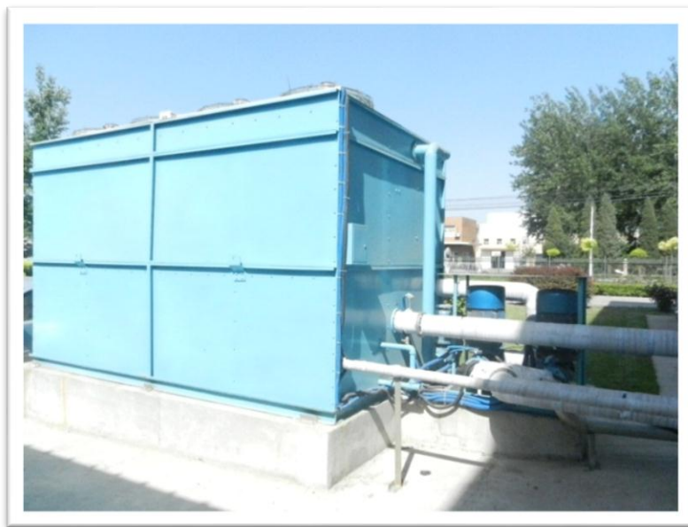
A machine enabling to reduce electricity consumption at Beijing
