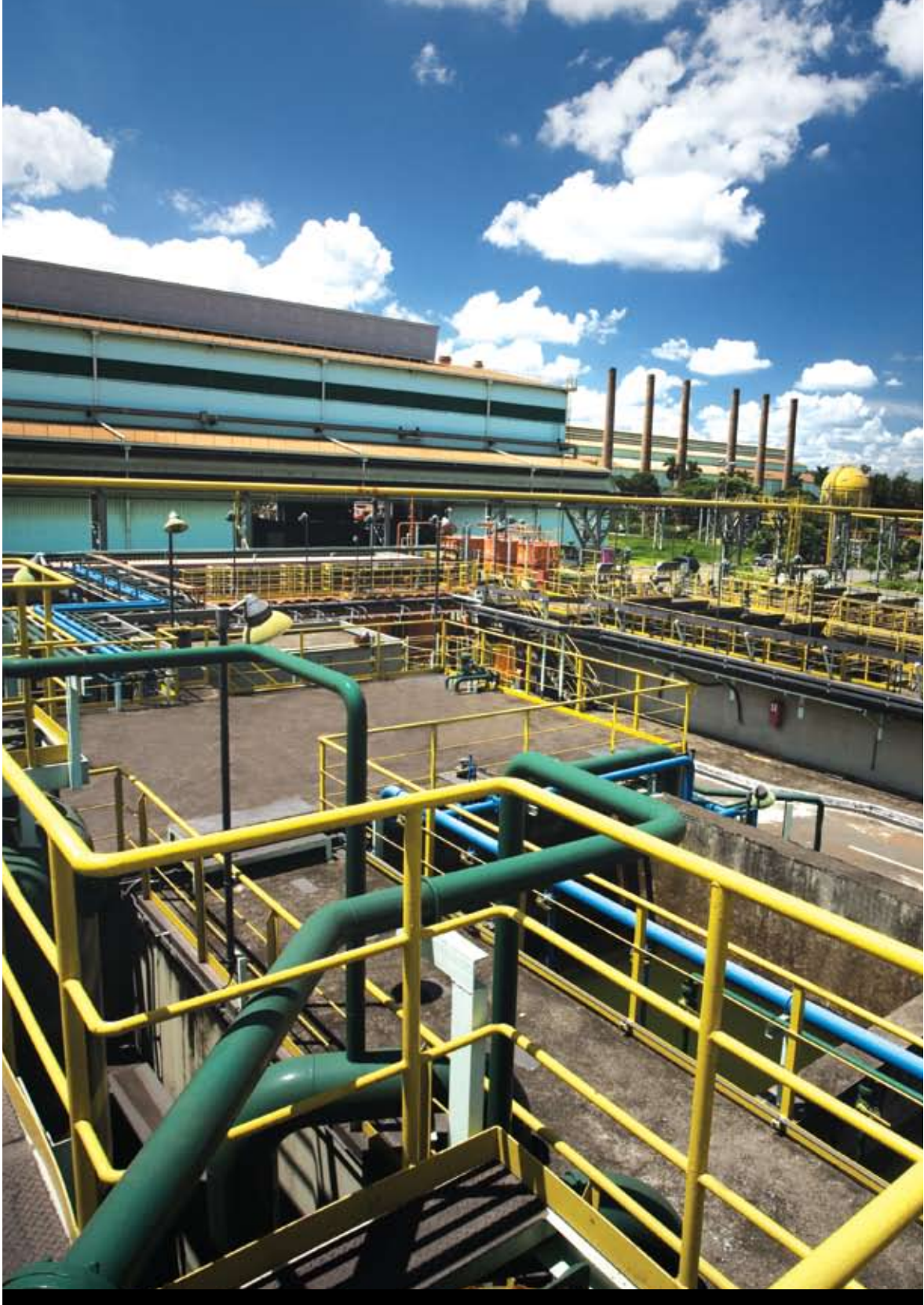
Effluent Treatment Station ( ETE ) at Unigal.
