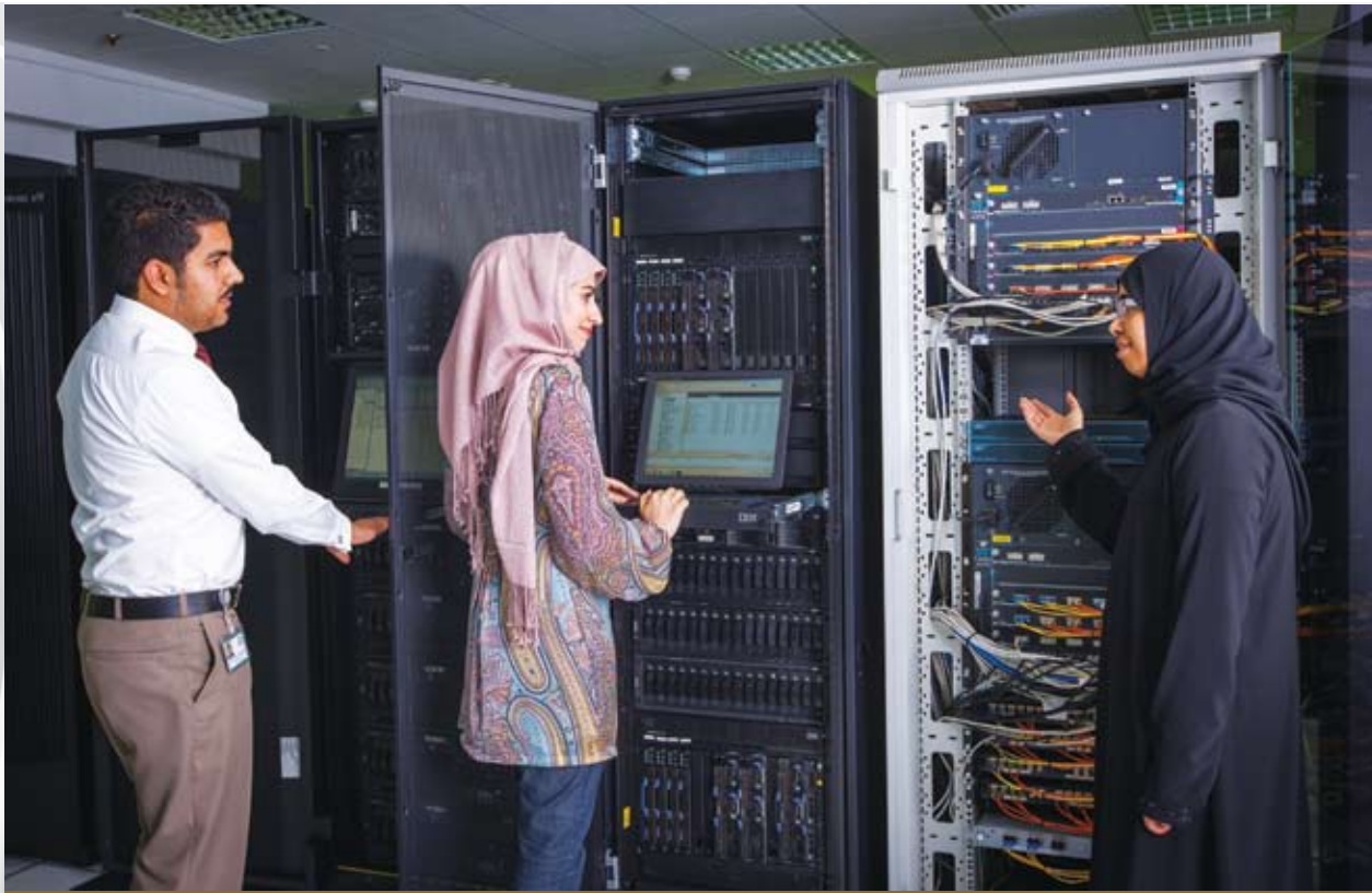
IT Server Room
