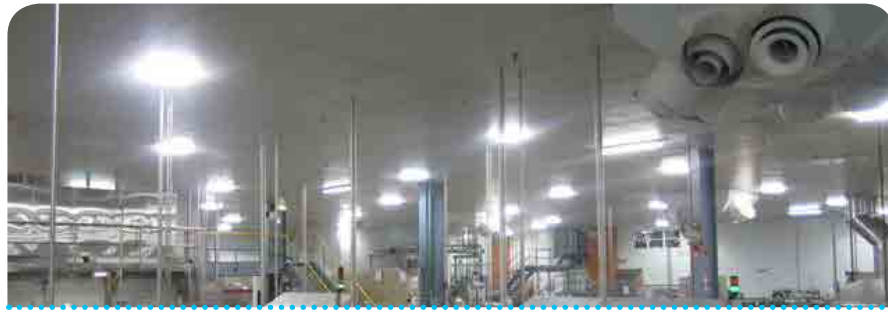
△ In Australia, high-efficiency lighting better illuminates the workspace while saving energy. The system uses programmable logic controllers and zoning to further reduce energy consumption.
