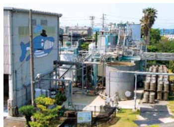
WARM project recycling equipment
