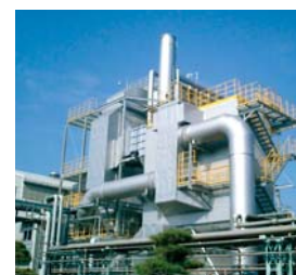
Biomass boiler at Shimonoseki Mitsui Chemicals
