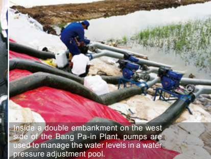
To accelerate the restart of operations, employees carry out maintenance activities despite pools of water remaining on the plant floor; Without power, employees labor amid hot and humid conditions.
