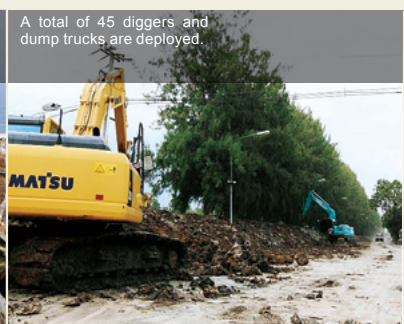
Earth embankments constructed with heavy machinery are covered with plastic sheets; Many employees cooperate due to the large scale of the embankments.
