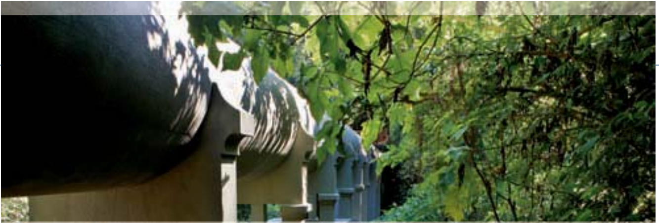
Water Treatment Plant feeder pipe - Alto Cotia
