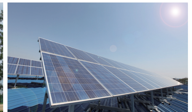
Namyang R&D Center solar electric system
