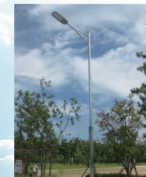
LED street lamps installed at Namyang R&D Center
