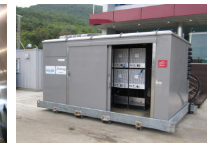
World's First Fuel Cell Generation Powered by Waste Resources
