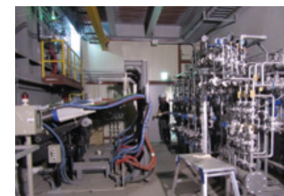
500kW Plasma Facility
