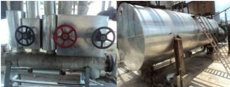
Lagging of steam valves and condensate tank
