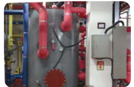
Geothermal Heating/AC Systems in Banghak Plant
