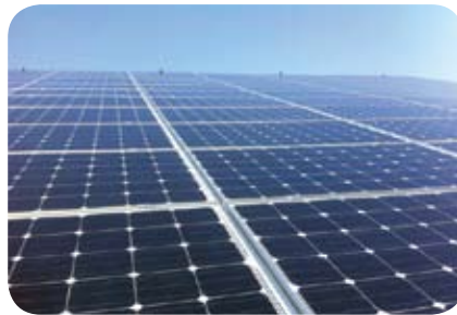
Taehwasan Solar Panels
