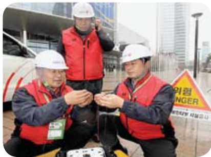
On March 23, kt staff connected optical cables near COEX in Samseong-dong, Gangnam-gu, Seoul
