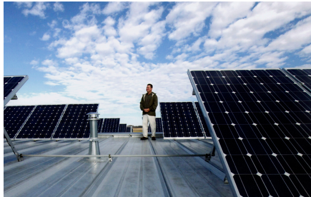
The solar array on the Promega Aviations Hangar is one of the largest statewide.
