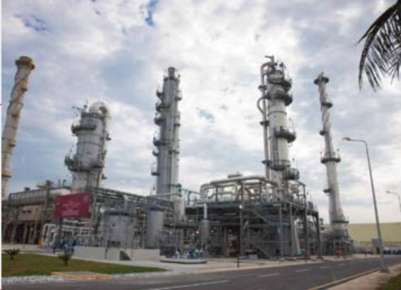
A view of carbon dioxide recovery unit
