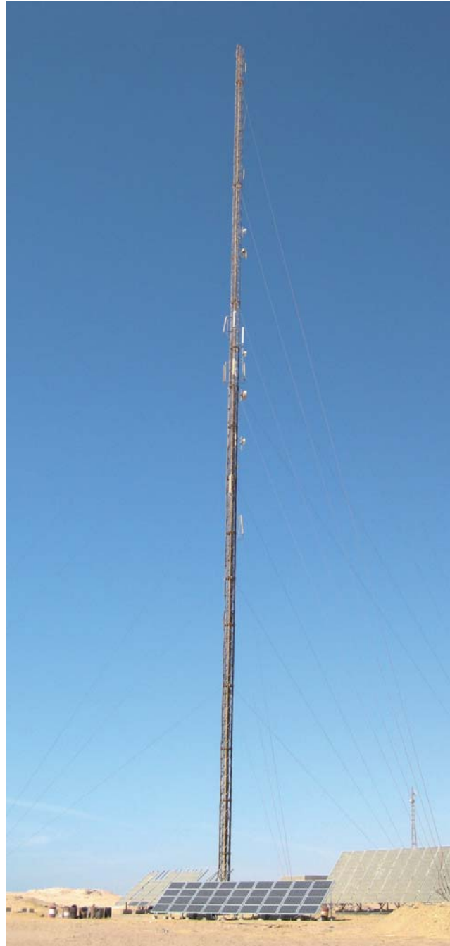
Base station equipped with a solar power system
