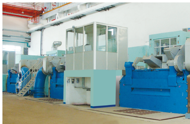
Intermediate frequency induction furnace
