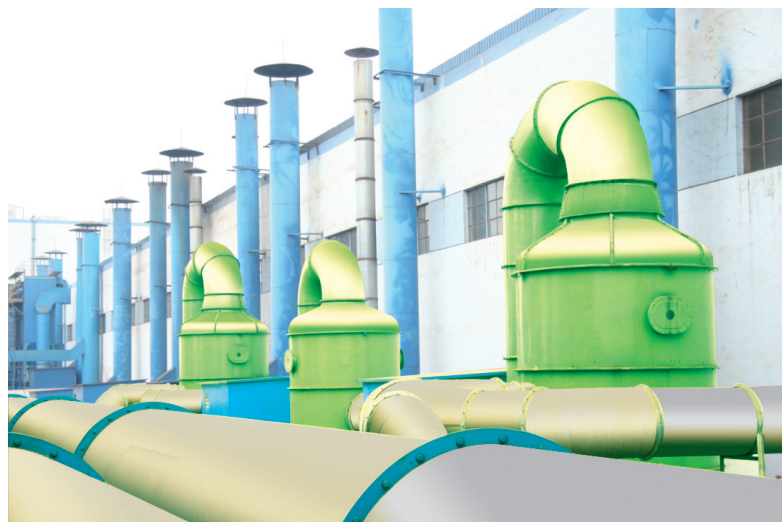
Scavenging towers in the casting center
