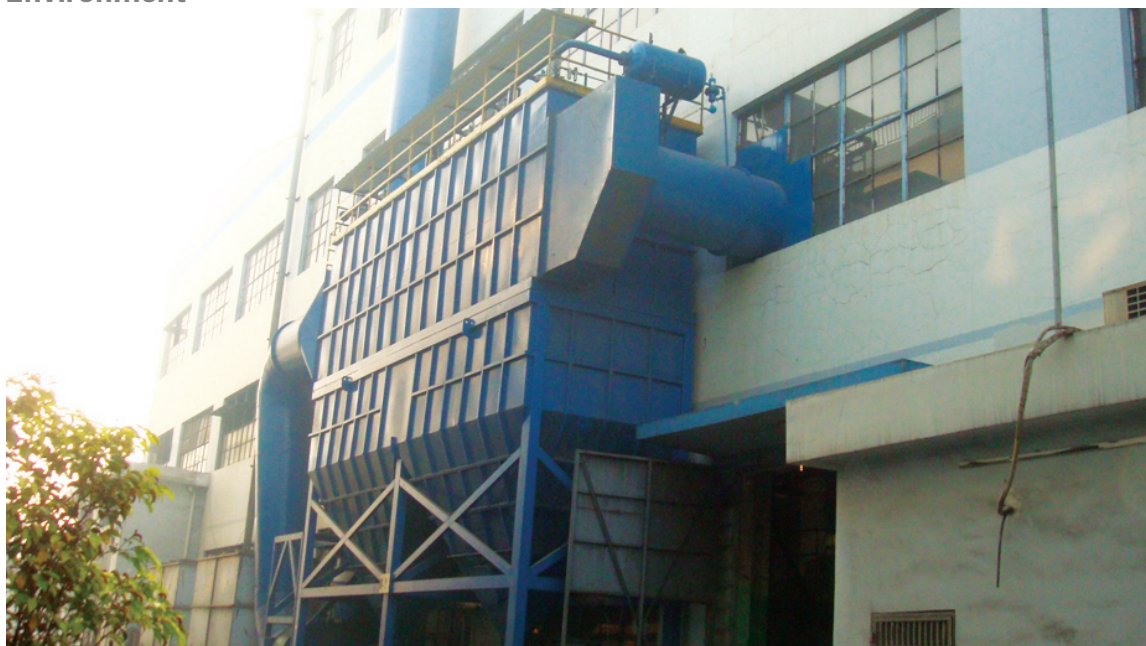
Flue gas treatment using intermediate frequency smelting furnace
