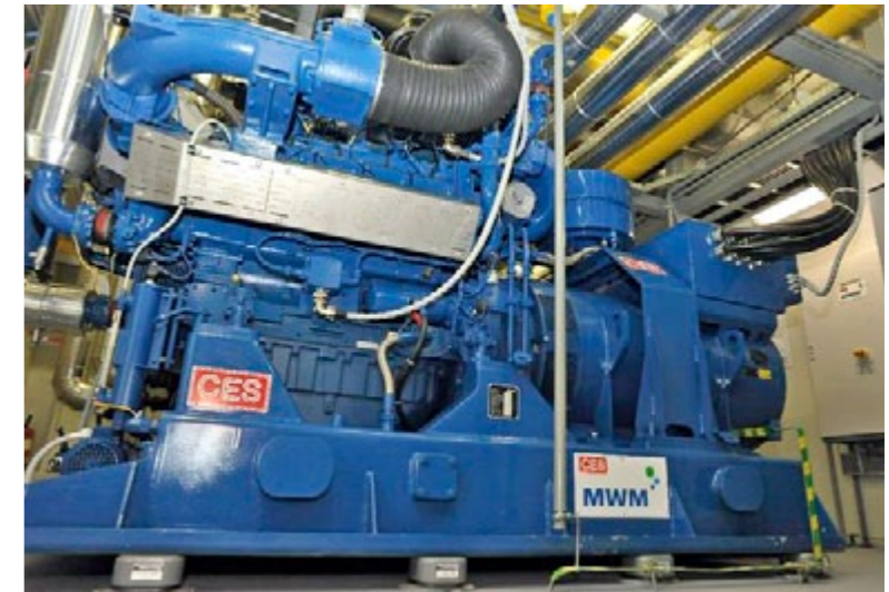
CHP system in MPEC Olsztyn]
