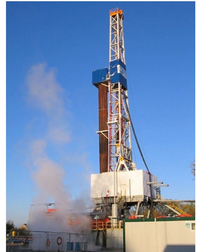
Geothermal drilling by PNiG Jasło – Landau project, as part of which a geothermal power plant was built in less than two years.
