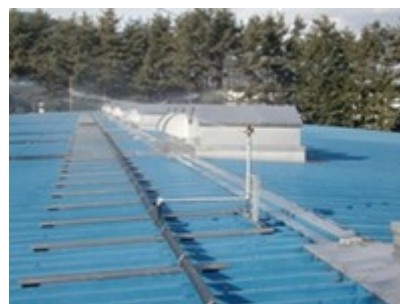
Test run status of circulating roof spray system
