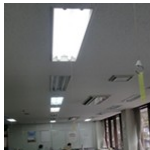
Thinning of lamp illumination and introduction of remote switch
