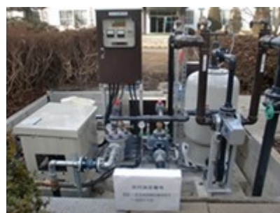
Pump for circulating water spray to building roofs
