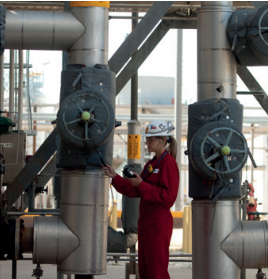
↑ Regular checks help maintain equipment at our Deer Park refinery in Texas, USA.
