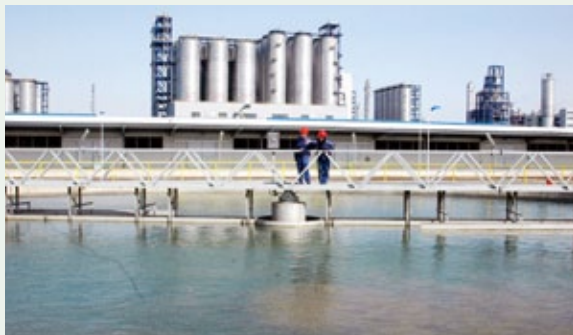
Waste water treatment plant, Sinopec Tianjin Company
