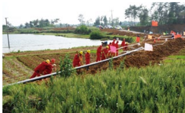
In May, in order to secure the gas supply to Beichuan, Sinopec South-west Petroleum Company started Deyang-to-Xinbeichuan gas pipeline project in Tashui Village, AN County, Mianyang City.
