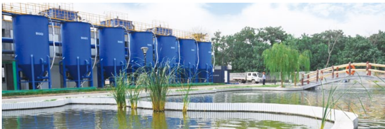
Waste Water Treatment Plant, Sinopec Qilu Company
