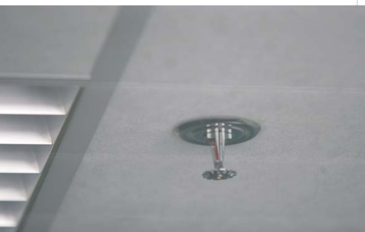
▼ In 2005, the dermo-cosmetic production site of Soual was equipped with a fire protection sprinkler system
