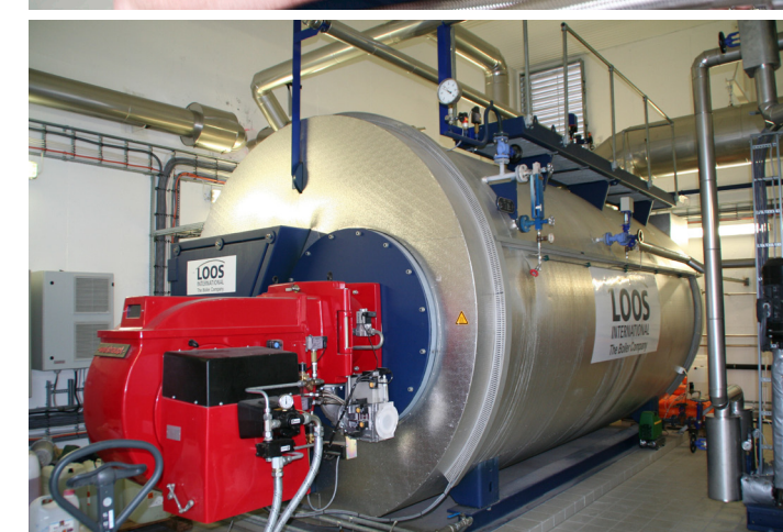
Top: Co-workers Mats Ivar Kjønnøy and Ståle Breivik monitor the production process at GC Rieber Oil’s production plant in Kristiansund, Norway. Above: The new steam boiler where bio diesel now has replaced fossil fuel.
