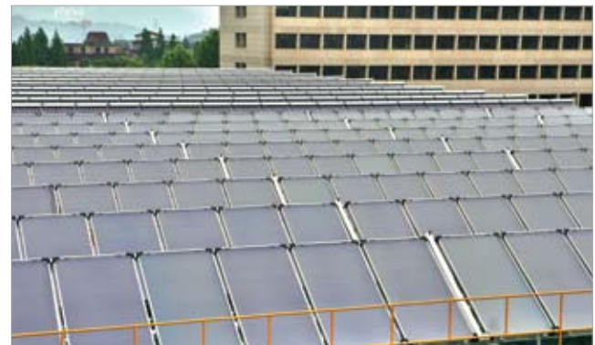
Building's rooftop solar light facilities
