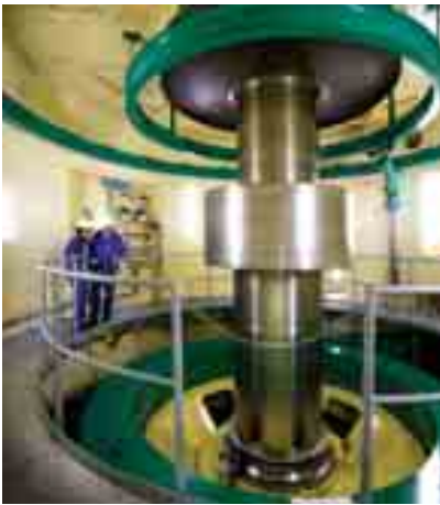
The motor driving the turbine at the Palmiet pumped storage scheme
