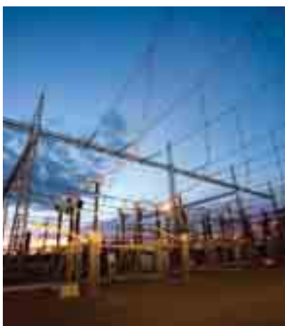
The high voltage yard at Apollo substation
