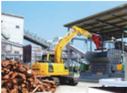
Inputting logging residues into a crushing machine (Niihama-Nishi thermal power plant)
