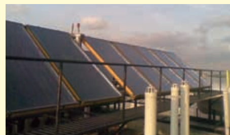
Hot water solar system
