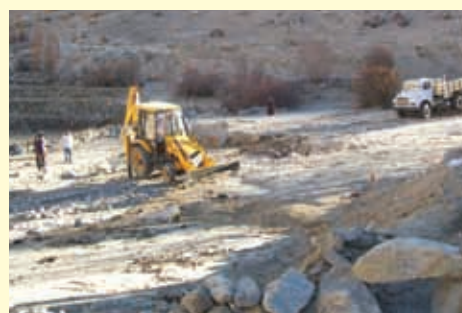
Debris removal work in progress at the affected village adopted by the Trust
