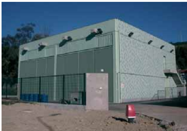
New HV/MV substation in Amadora
