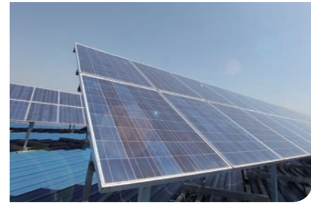
A solar panel system on the rooftop of R&D Museum at the Namyang R&D Center
