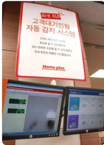
'Automatic customer queuing system' installed in the Yeongdeungpo store and Jamsil store reduce customer wait time and improve the efficiency of cashiers.
