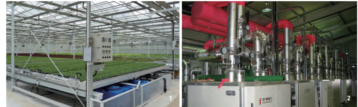
1,2 Young leaf cultivating facility of Pulmuone Farm and Heating and Cooling system using geothermal heat.
