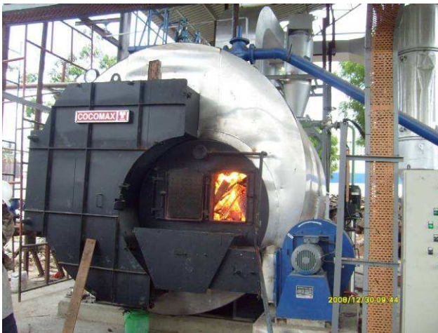
One of the newly commissioned biomass boilers.
