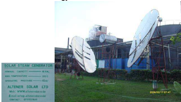
Pilot Solar Plant.
