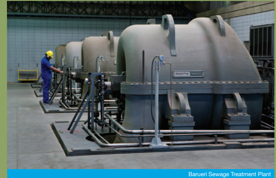
Barueri Sewage Treatment Plant
