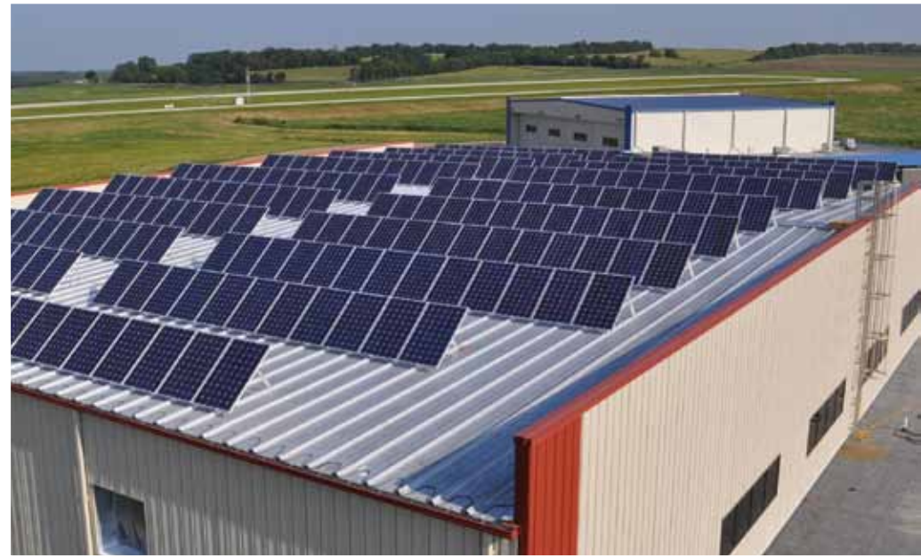
The solar array on the Promega Aviations Hangar is one of the largest statewide.
