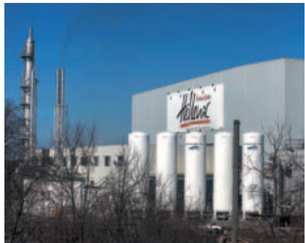
On-site Combined Heat and Power (CHP) units are now operational at four bottling plants; a further five are due to become operational in 2011.
