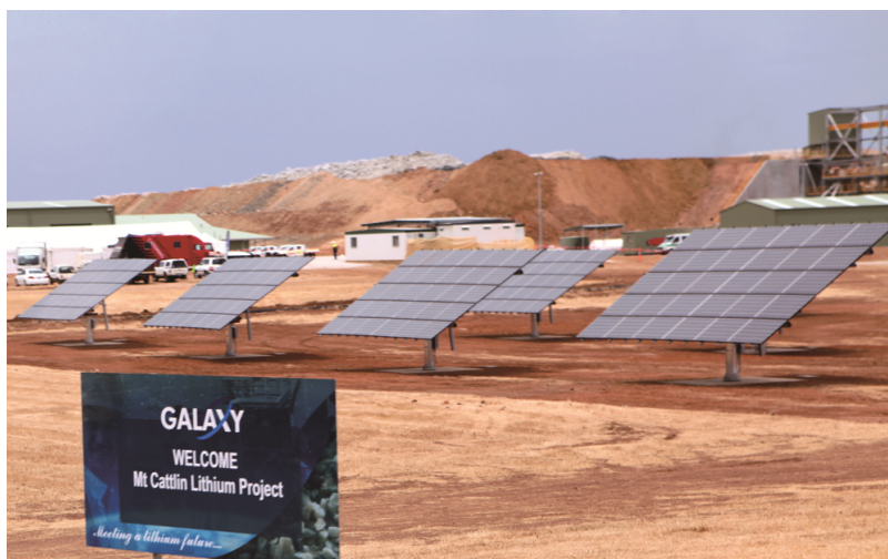
The Solar panels power system of Cattlin spodumene lithium mine
