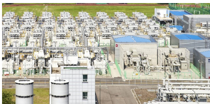
KOSPO | Shinincheon Bitdream Hydrogen Fuel Cell Power Plant
