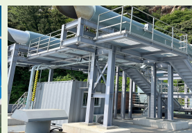
KEPCO, Air Pollution Reduction Facilities (Jeodong, Ulleungdo)
