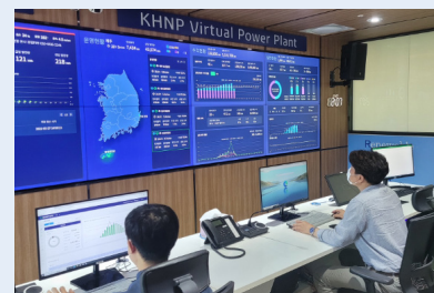
The Renewable Energy Control Center
