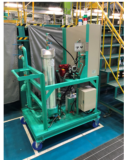
Oil Purification System
