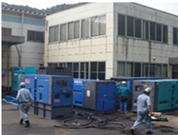
Disaster recovery support (lending electric generators)
