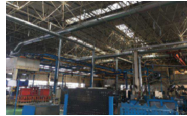
An example of measures to meet regulations in China (Daikyo Machinery Shandong Co., Ltd.: Installation of a welding fume dust collector and exhaust air ducts)
