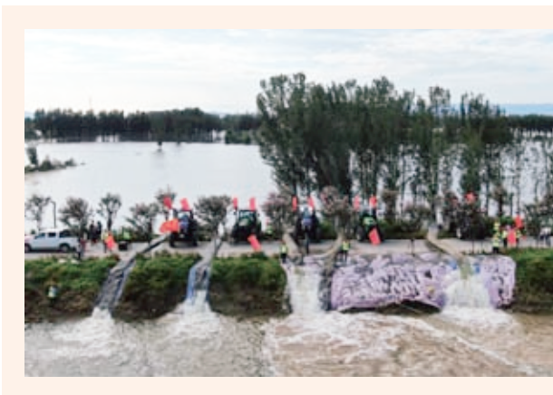
调集先进的抽排水与发电设备 Assisting flood control and disaster relief in Henan
