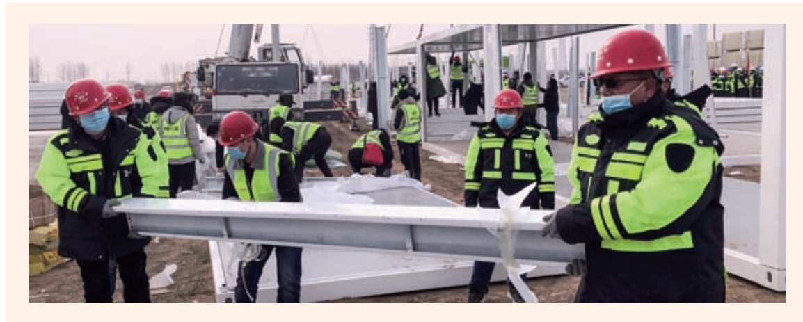
石家庄黄庄公寓隔离点援建人员搬运板房材料 Transporting materials for construction
