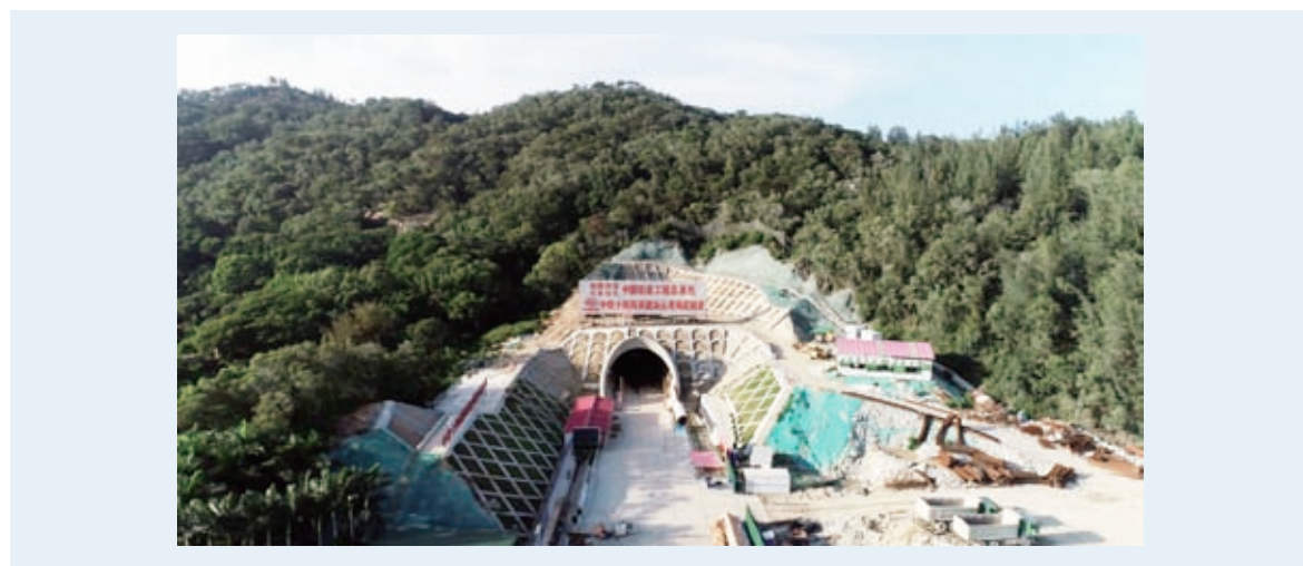
汕汕铁路汕头湾海底隧道顺利掘进千米 Shantou Bay Subsea Tunnel of Shantou-Shanwei High-speed Railway
