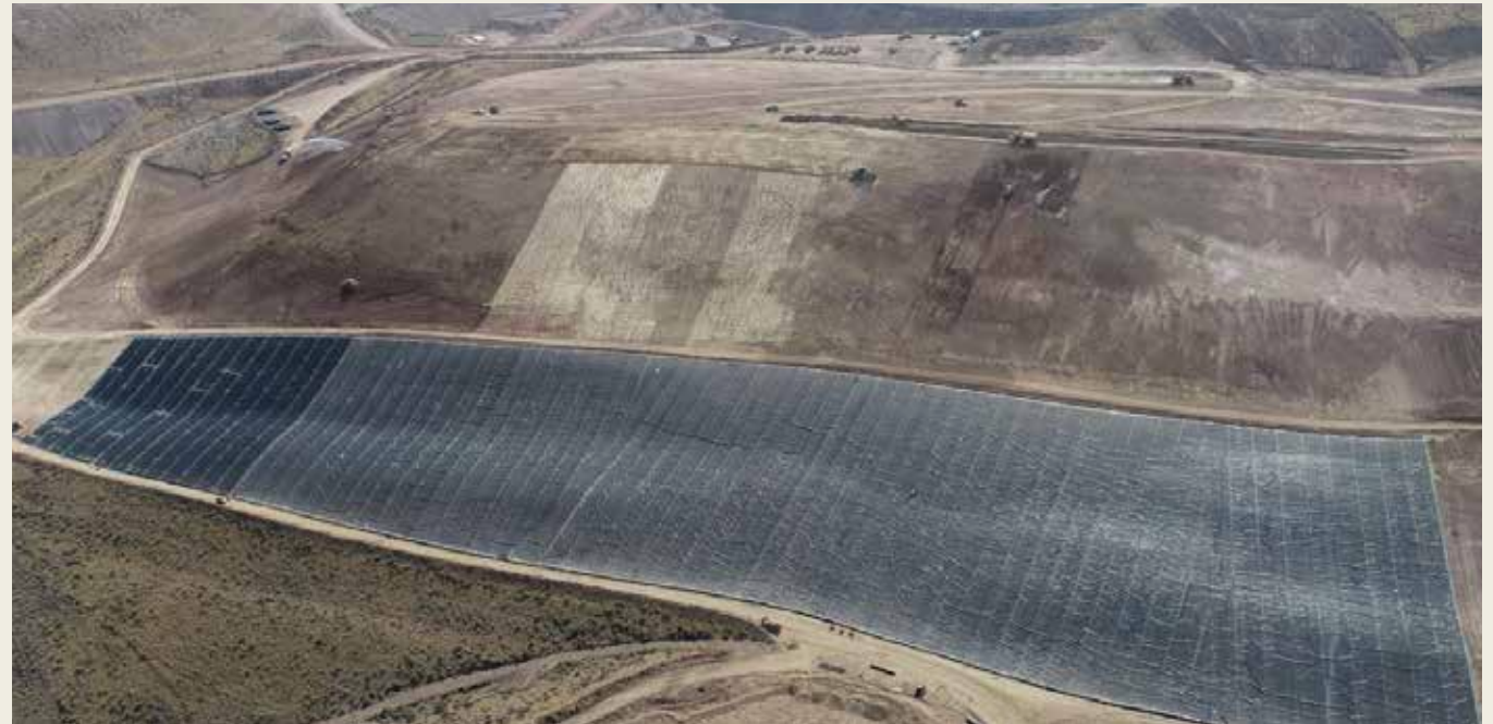
Rehabilitation activities at Rain, including the laying of the HDPE liner before the geotextile, cover material and topsoil deployment - NGM, USA.
