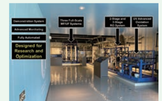
The demonstration system at the Las Virgenes Municipal Water District
