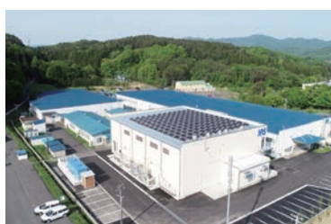
Solar power generating station (roof top)(Tohoku Hirose Electric)
