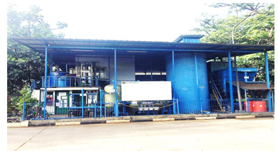
Komatsu Indonesia's wastewater recycling facility
