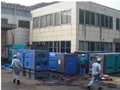
Disaster recovery support (lending electric generators)
