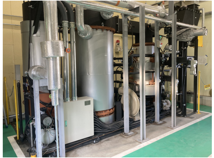
Ibaraki Plant biomass boiler
