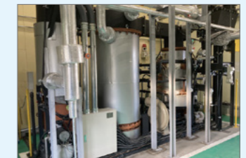
Biomass boiler at Ibaraki Plant
